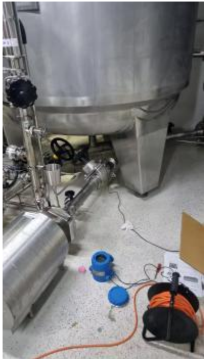
In Kuwait, WFI(Water for Injection) tank
