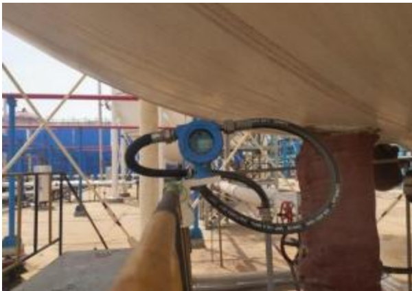
In China, LPG spherical tank/Skid package
